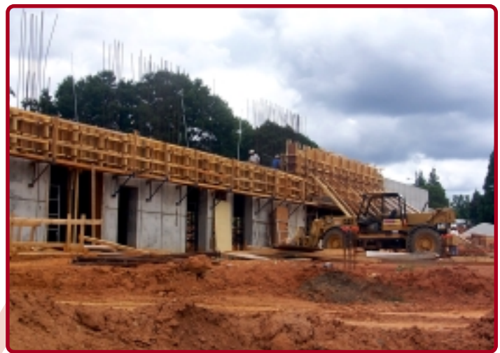
Above: Construction of the McSwain Education Center is well underway and is scheduled for completion in March 2002.
