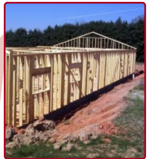
Above: The staff/volunteer building is on target for an early fall completion date.
