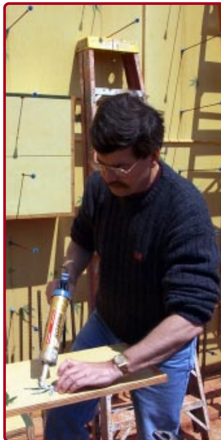
Above: Bob Lyons pushed up his sleeves to help build the McSwain Education Center along with several other volunteers and staff members.
