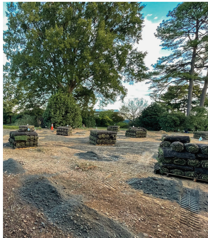
Forty-seven pallets of fresh sod ready to be installed on the Gathering Lawn.
